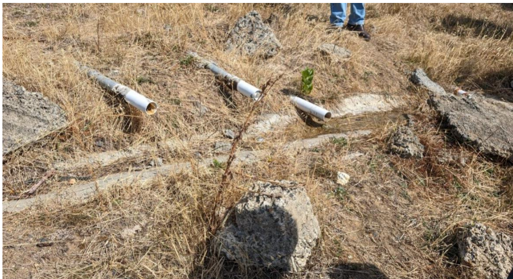
Figure 5: Array 4 outflow point of horizontal drains, minor flow only (image: pitt&sherry, 19th March 2024).
