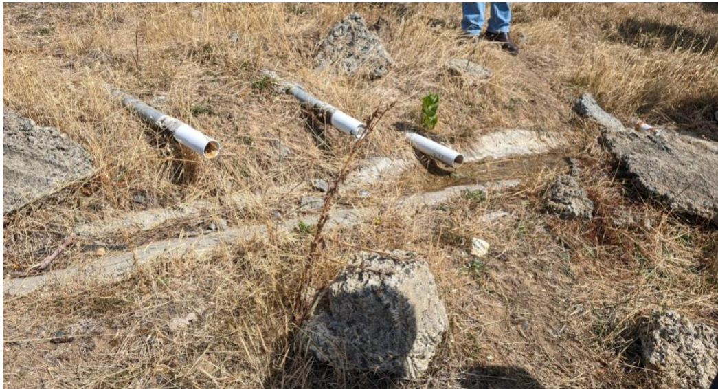
Figure 4: Array 4 outflow point of horizontal drains, minor flow only (image: pitt&sherry, 19th March 2024).
