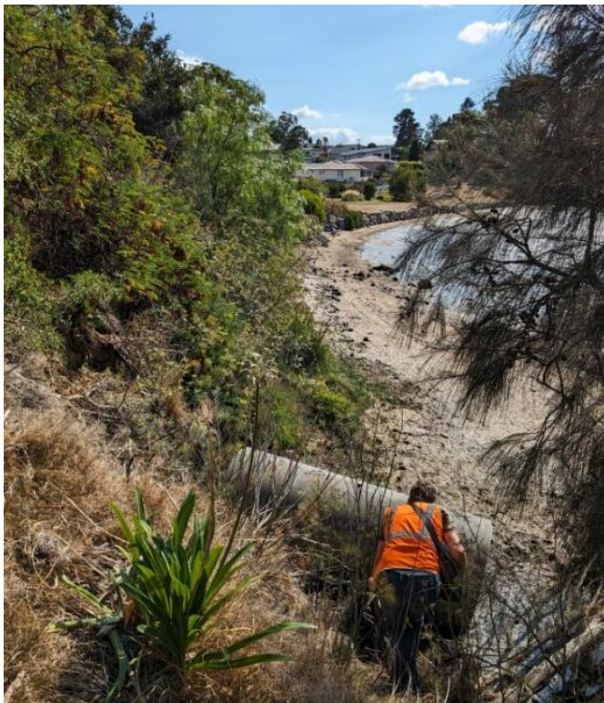
Figure 7: Disconnected stormwater outfall pipe; Casuarina landslip area
