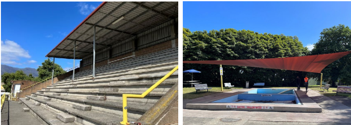
Image 13: Outdated grand stand with structural issues and open air toddler pools not suitable during colder days.
