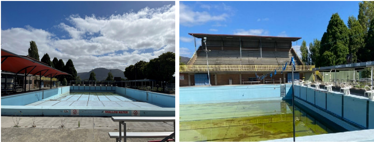
Image 12: Drained pool with significant issues.
